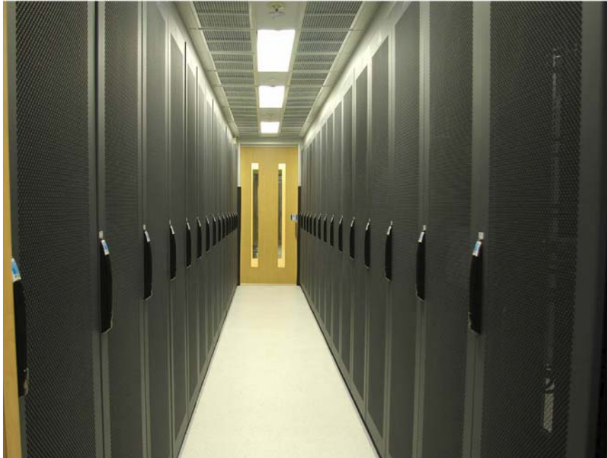
Figure 2) Cold room tunnel.
